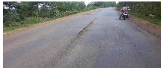
Figure 2.2. Pavement defects in the study area
