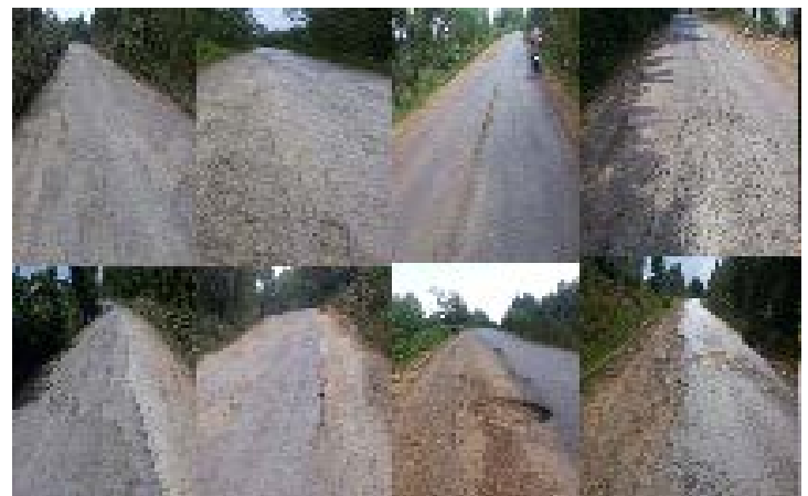
Figure 1.1 Current Condition on some Sections of Yebu-Agaro Road
